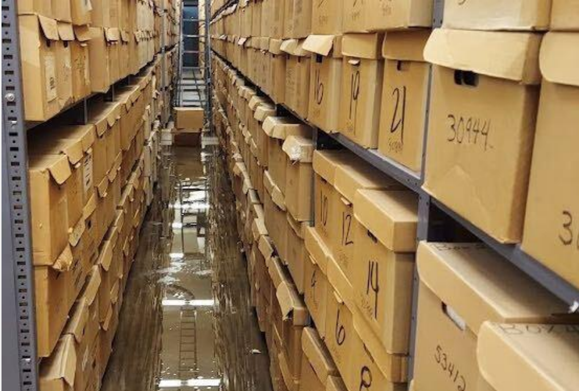
Photograph of flood in Colorado State Archives stacks, December 27, 2022, provided to Colorado Public Radio by the Colorado Department of Personnel and Administration
